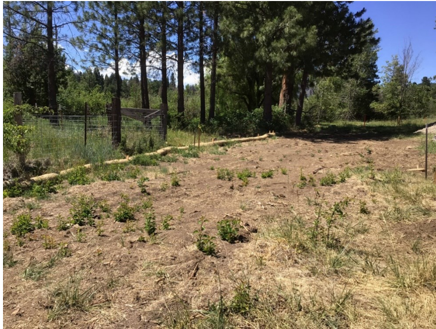
Photo 5: SWPPP BMPs (fiber rolls) were placed along northern site boundary in accordance with APM WQ-1
